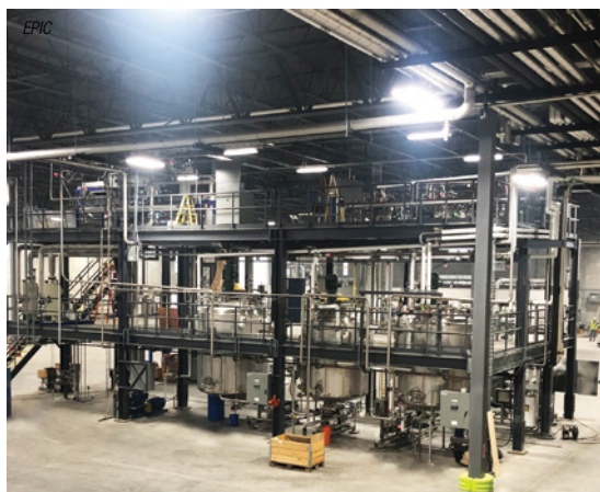
FIGURE 4. Modular construction firms typically have project managers, procurement, project designers and engineers in various disciplines on site, so anything that needs to be adjusted can be handled in the fastest and most seamless way, which means there is a significant reduction in time to market. Shown here is a turnkey modular system that EPIC designed and built for installation at a customer's facility
